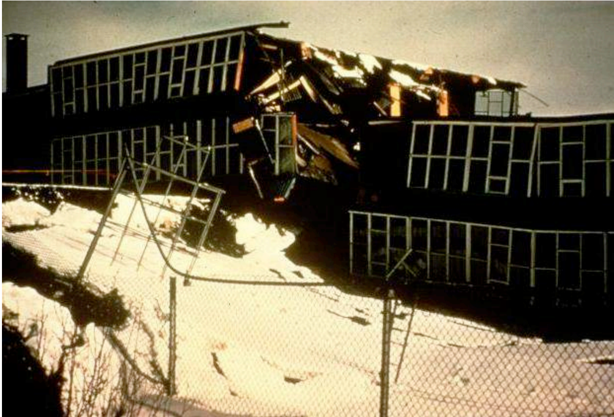
Figure 22f. An Anchorage area school cut in two by a fault scarp with offset equal to about one story of the school. The greatest loss of life in Port au Prince was when the floors of large public buildings collapsed in on each other. In contrast, this school is almost intact except right in the exact fault zone. Notice that almost all lines in the school are almost perfectly straight, including the roof line that has been sheared by the fault. This school in Anchorage performed superbly - kids would have been safe in the entire school except for about twenty feet right in the fault zone. (Photo from Wikipedia)
