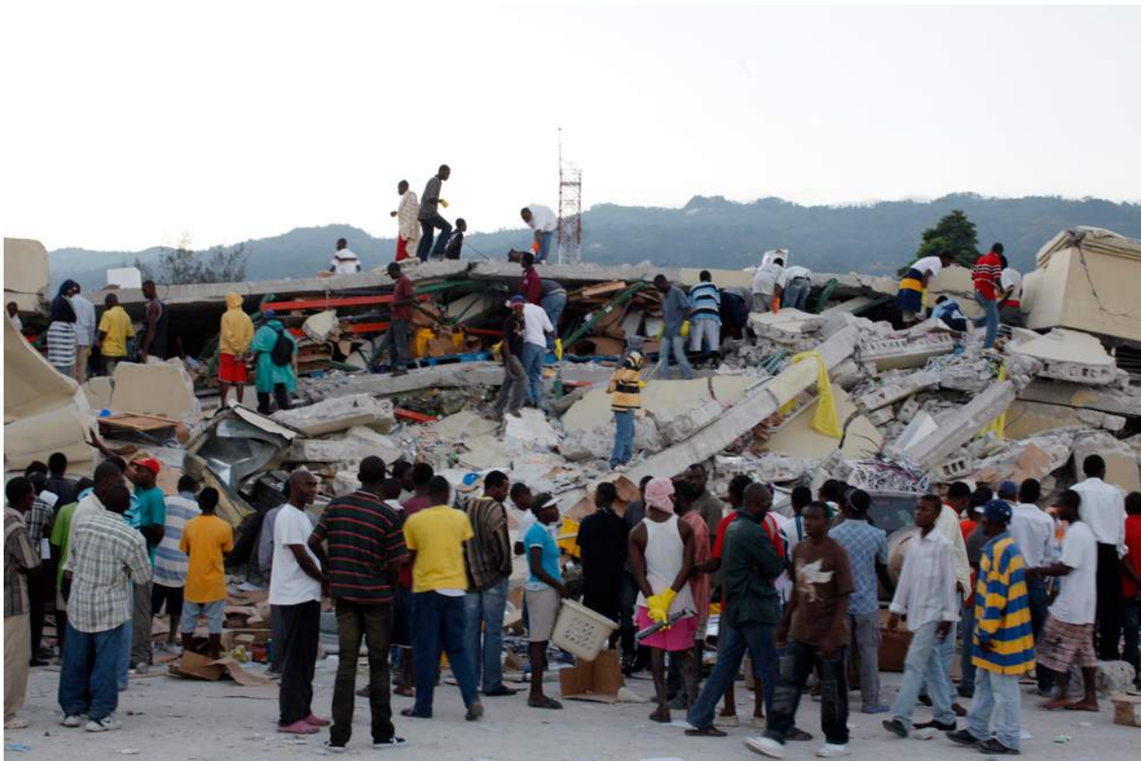
Figure 22d. Every thing bad shows here. The roof and floors are flat slabs instead of engineered designs with integrated beams to give it depth but not unneeded weight. Good floor designs look like a worms-eye view of a waffle from underneath. Sections of under-fit concrete block walls appear to have been the main vertical support. No rebar is showing.
