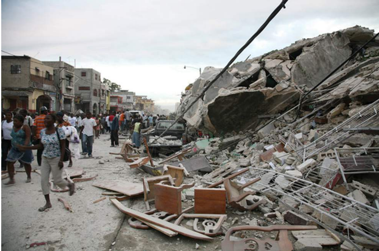
Figure 22e. Port au Prince. What a difference between this and the Anchorage school. This Port au Prince commercial building has gone past the stage of shear cracks, past the stage of floors collapsing on floors, and has disintegrated to rubble. No one could have lived through it.
