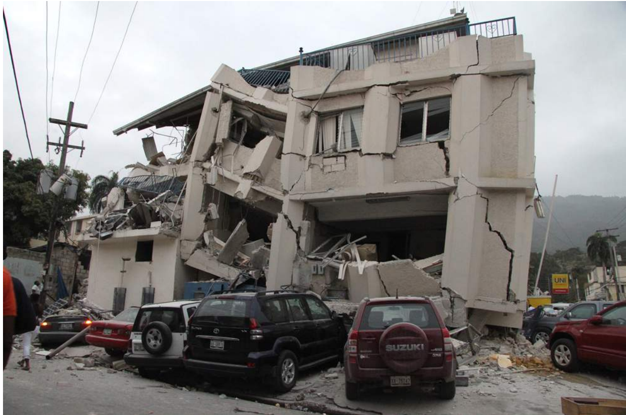
Figure 22c . Sometimes one set of shears dominates and the building begins to collapse sideways. Note the large intact segments of corner columns. They probably prevented, but barely, total collapse.
